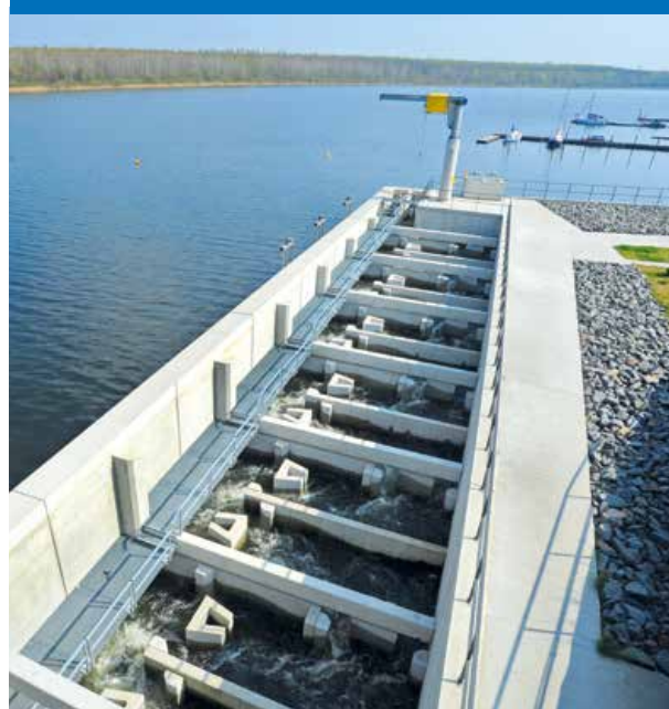
Fish ladder at river Mulde reservoir
